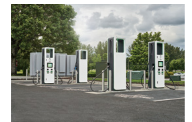
EV rapid charging stations made by Signet
