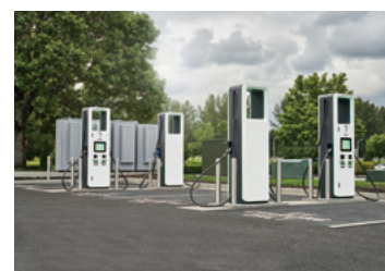
EV rapid charging stations made by Signet
