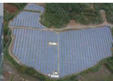
Itako Mega-solar (Ibaraki Prefecture)
